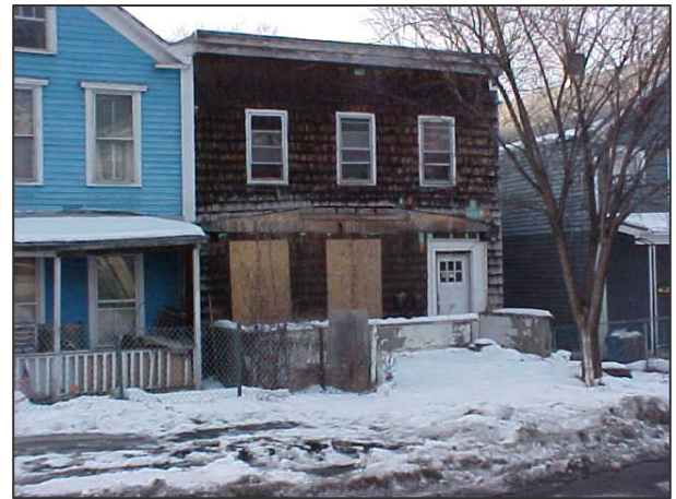
Deteriorated houses, such as the brown building on the right, have a negative impact on the surrounding neighborhood
